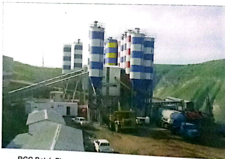
RCC Batch Plant, aggregate conveyors, and cooling units.
