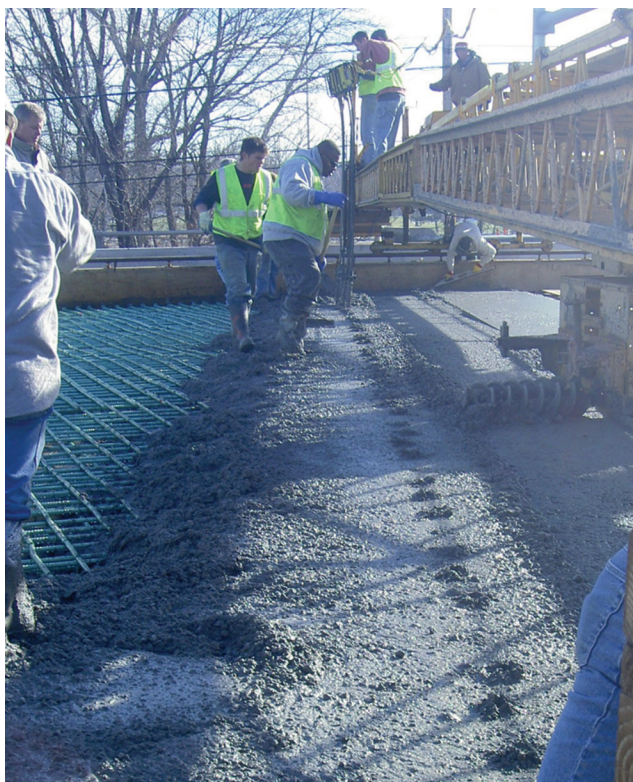
Fig. 4—Holes left by vibrators on LC-HPC-14 Placement 1 (McLeod et al. 2009).
